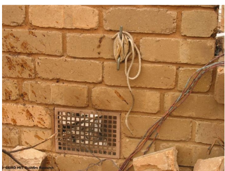
Exposed vents may allow entry of sparks and embers.
