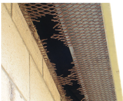
Gaps in eaves may allow entry of sparks and embers.
