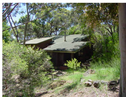
Trees overhanging your house will drop dead leaves and twigs into your gutters.
